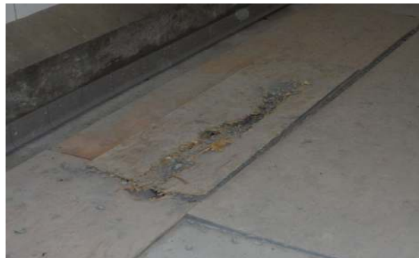
Deficient Hole Cover
