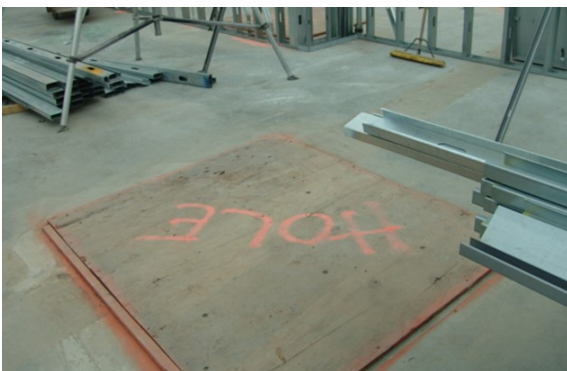
Adequate Hole Cover
